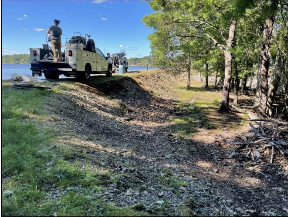
Photo No. 5.: Downstream slope of the dam embankment from near the right abutment looking left.
