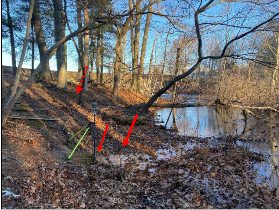
Photo No. 11.: Seepage at the downstream toe of the native terrain after drawdown (solid arrows). The dashed arrow indicates the approximate location of the seepage from the slope during normal pool levels (see Photo No. 9)
