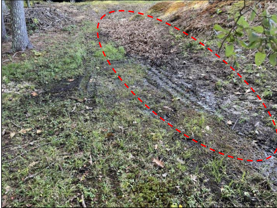
Photo No. 7.: Saturated area along the downstream toe of the dam (atop the native terrain) during normal pool (looking right).
