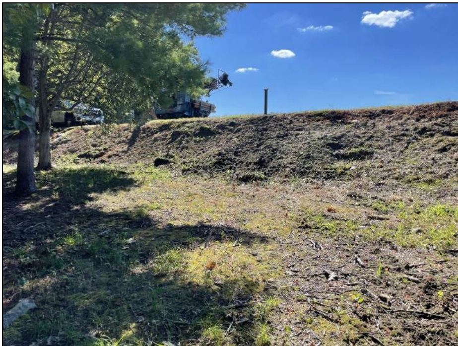
Photo No. 6.: Overview of the study area downstream slope from the toe of the dam looking right. Note the steep slope and uneven surface throughout.
