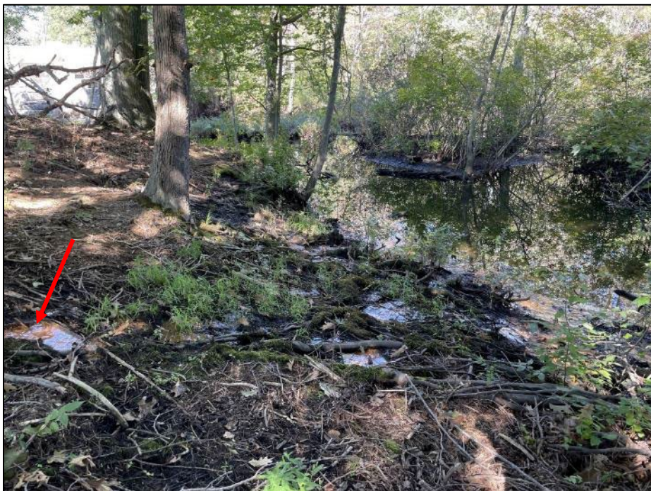
Photo No. 8.: Active seepage breakout with iron oxide staining along the downstream toe of the native terrain.
