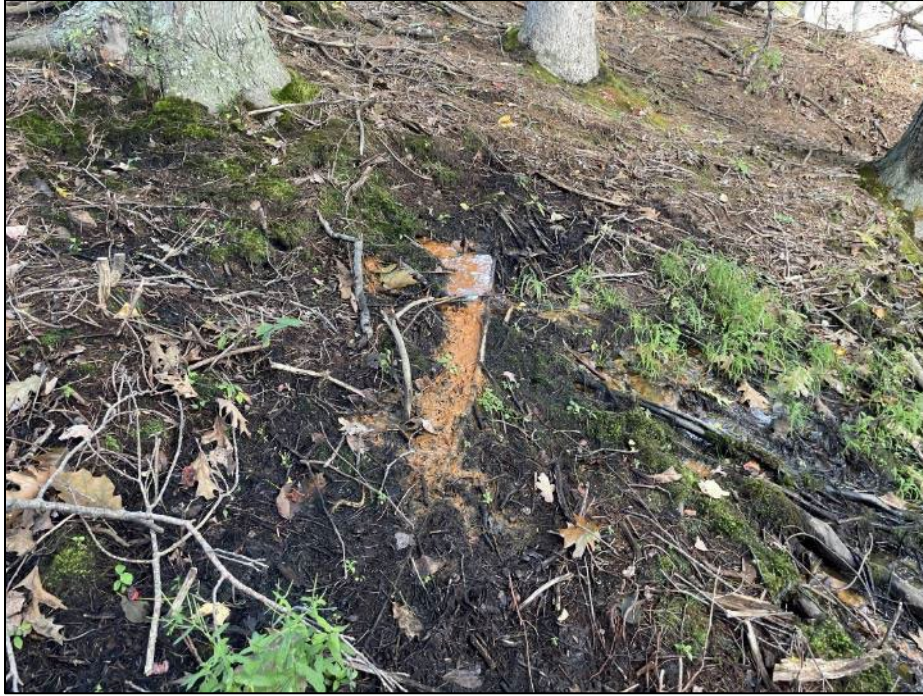
Photo No. 9.: Closer view of the seepage at the downstream toe of the native terrain.
