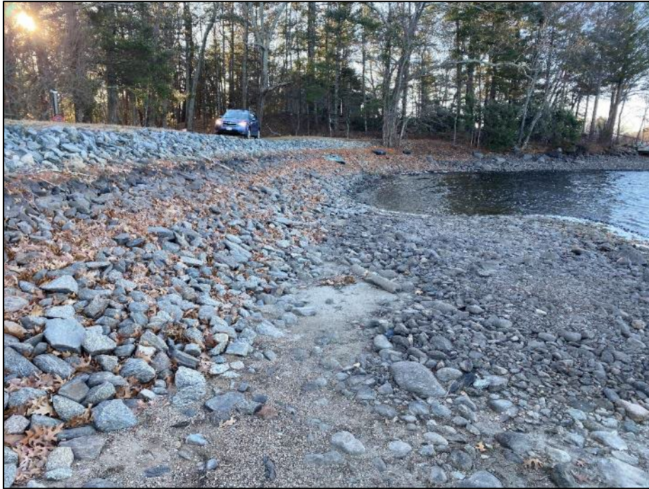
Photo No. 3.: Upstream view of the study area from the bedrock outcrop looking right after drawdown of the impoundment.
